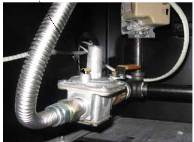
Broiler Pressure Regulator (close-up view)
